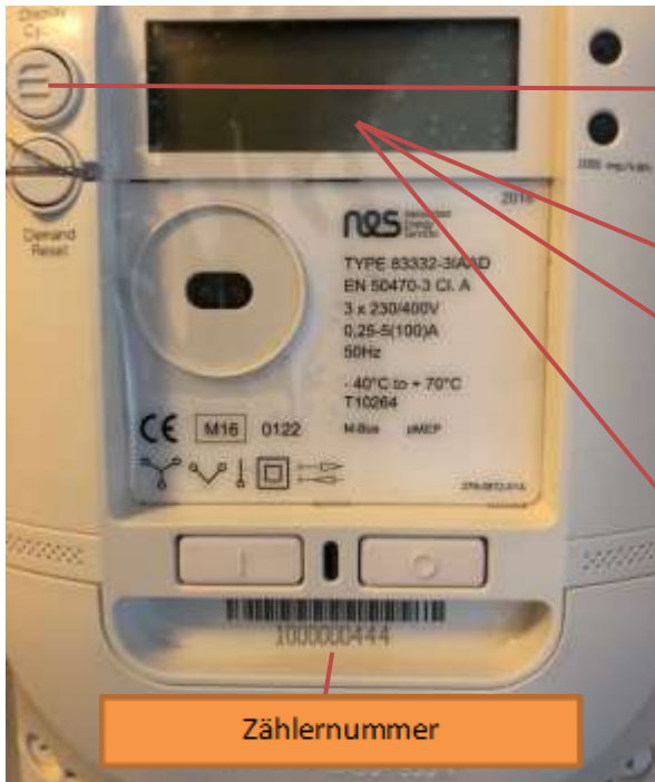
Zähler NES Networked Energy Services
